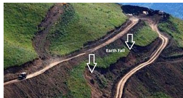
Figure 9) Soil mass movements in soil-type road trenches.
