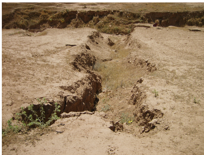
Figure 2 A sample of the gullies in Dehloran region
